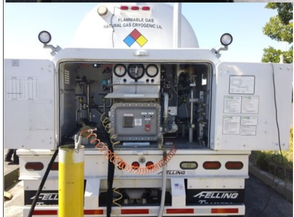
An Ammonia Fueling station could be similar to this compressed natural gas filling station in Sacramento, California. Specially designed nozzle for easily and safely dispensing fuel (top). Portable fueling station mounted on a Felling Trailer (Sauk Center, MN) platform (bottom).
