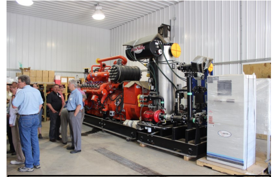
Visitors examine one of the generators at Riverview Dairy's 1.5 MW anaerobic digestion system in Stevens County
