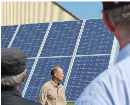
Bruce Freske of the US Fish and Wildlife Service discusses the 20 KW solar electric system they are using at their Morris Office
