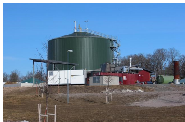
Lövesta research farm anaerobic digester- capable of 500 kw of electrical production and a significant portion of building heating.
